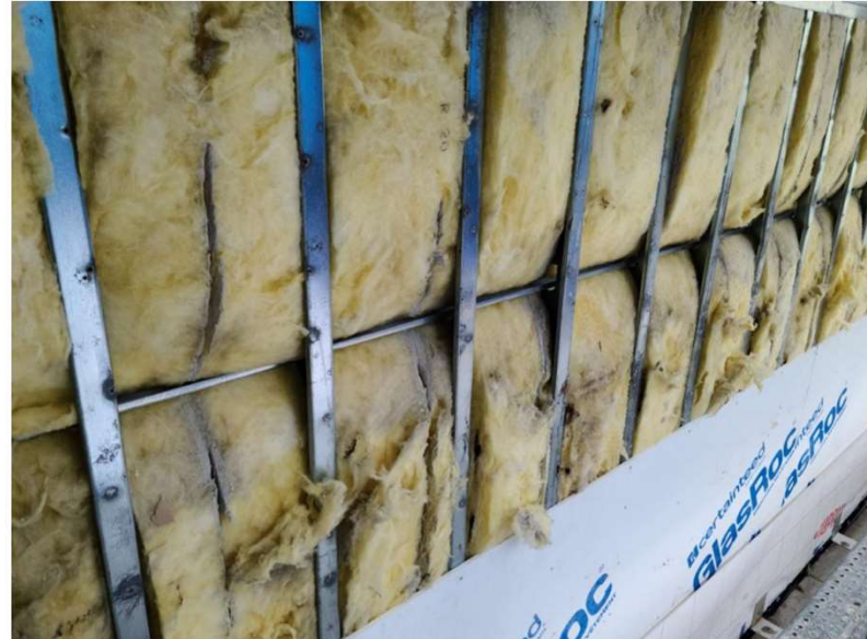
Photo 7.11: Add batt insulation where original insulation wraps around stud bracing leaving gaps in the stud cavity
