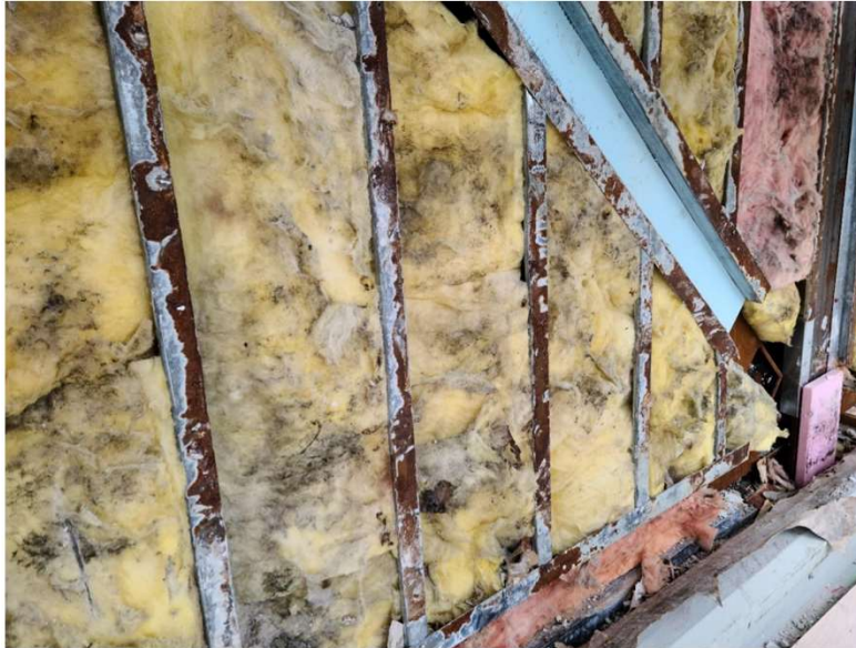
2.2 View of corrosion on surface of steel studs. Structural steel is also exhibiting some surface corrosion. Coping blocks on top of the concrete masonry are unsecured and require further review by the structural engineer.
